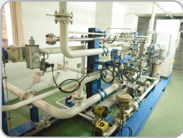
Nitrogen producing station - firm «Linde» (Germany)
